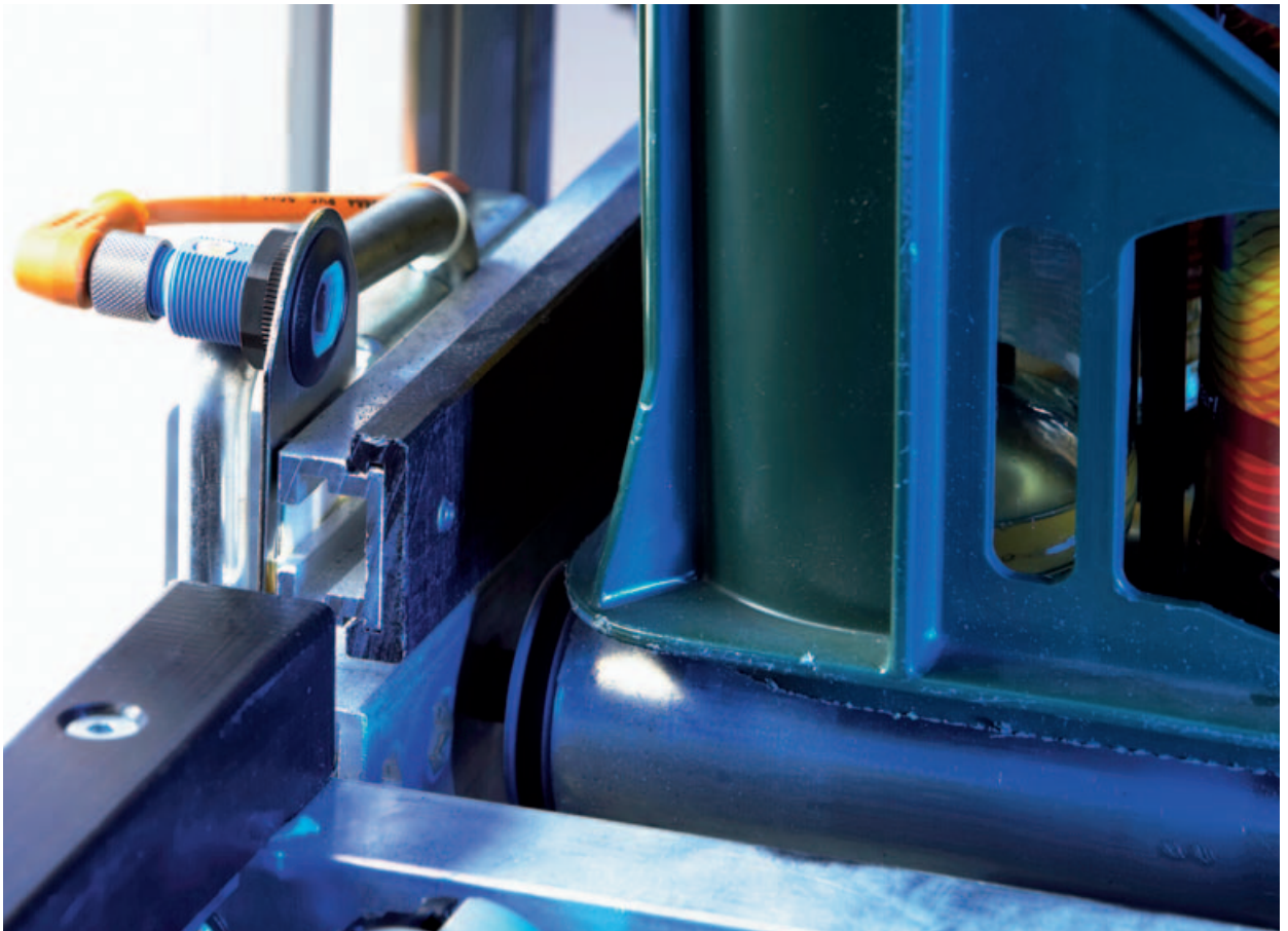
► Backup control with an MHL 15 photoelectric reflex switch in beverages picking.
