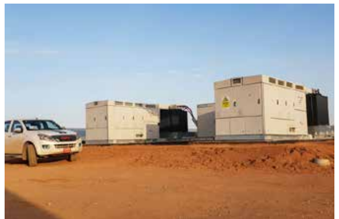
EGYPT Alcazar, 283 MW HEMK+ TWIN SKID
