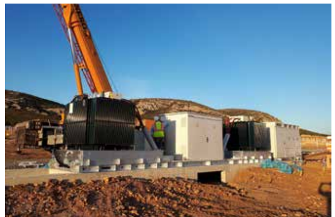
SPAIN La Nava, 46 MW HEMK + TWIN SKID
