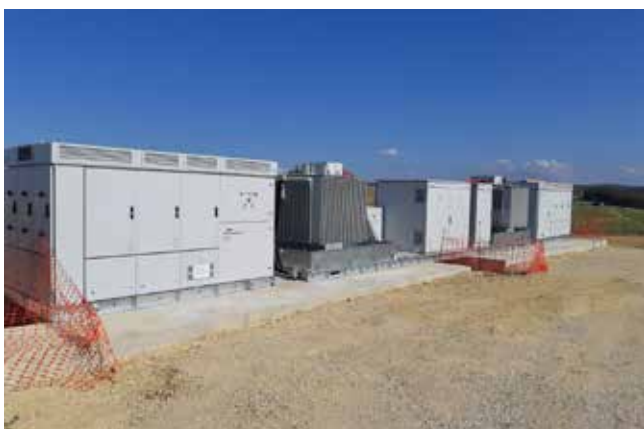
SPAIN Guillena, 105 MW HEMK+ TWIN SKID
