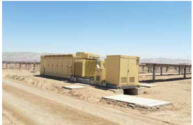
CHILE Uribe, 50 MW HEC PLUS + MV SKID
