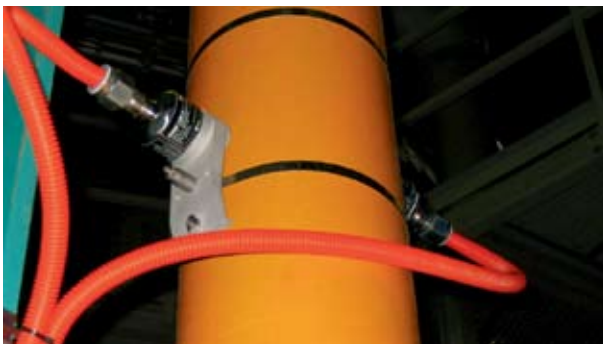
Quench water flow measurement on a rubber lined pipe
