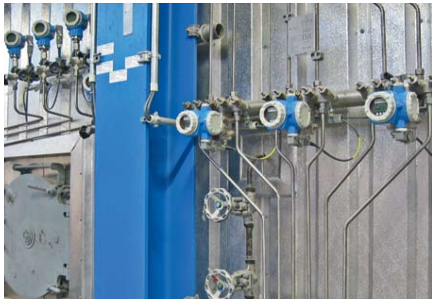
dp level measurement of the steam drum with Deltabar S PMD75
