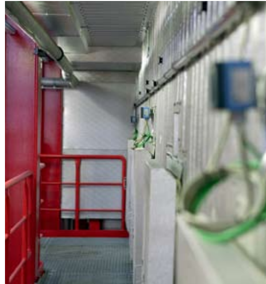
Temperature measurement at the superheater, horizontal flue
