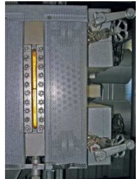
Visual steam drum level control through a sight glass
