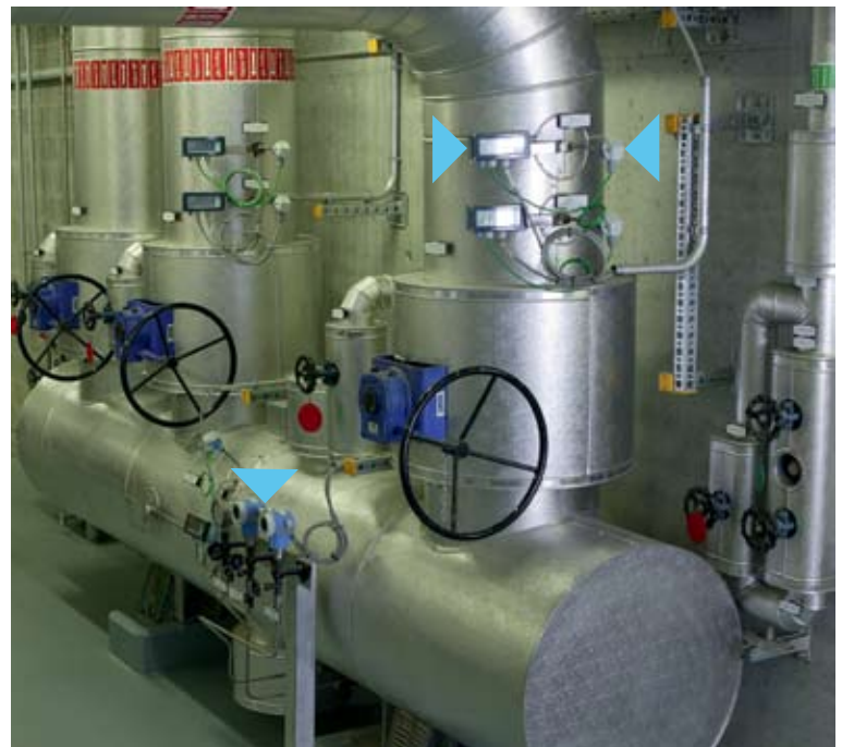
Redundant pressure monitoring at the high and medium pressure distributor and a redundant temperature monitoring in the main pressure pipe by TC15 and the RIT261 display.
