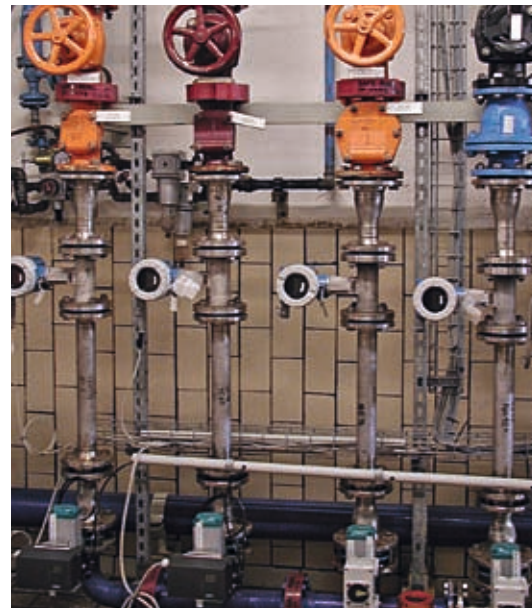
Prowirl monitors the flow volume of the fully desalinated water
