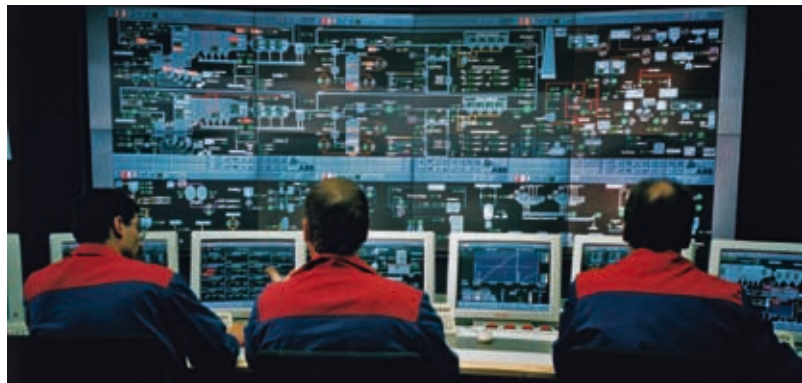
Control room of a modern power plant
