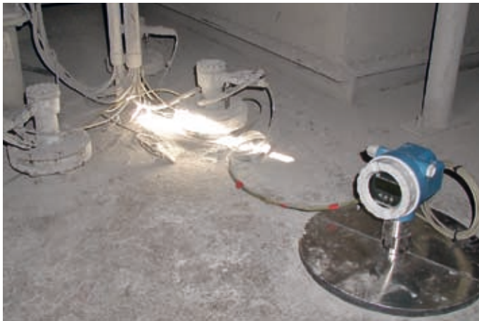
Levelflex monitors level and Soliphant measures maximum limit in the lime silo
