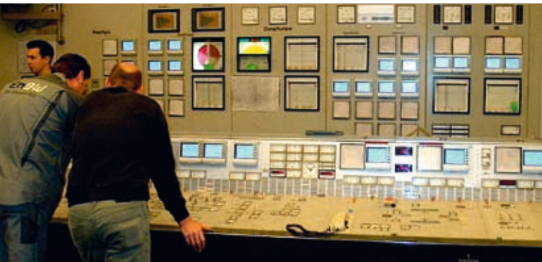
Ecograph/Memograph data recorders installed in a control room
