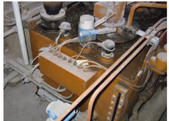
Level measurement in an hydraulic oil tank
